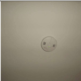
12/12/2014 Basement CO smoke alarm DSC03797 site 809 Basement CO Smoke alarm.JPG
