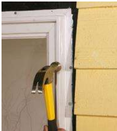
Adding too many nails to the nailing flanges is a common mistake.
