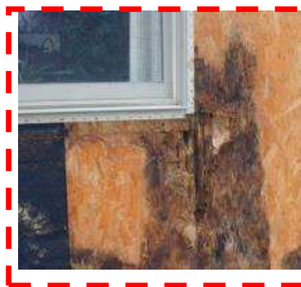
Typical pattern of rot deterioration of wood sheathing and stud framing in wall area below improperly installed windows
