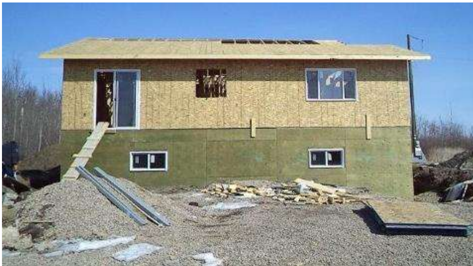
Windows installed directly into the wood framed wall without membrane wrap of the rough opening in the wall
