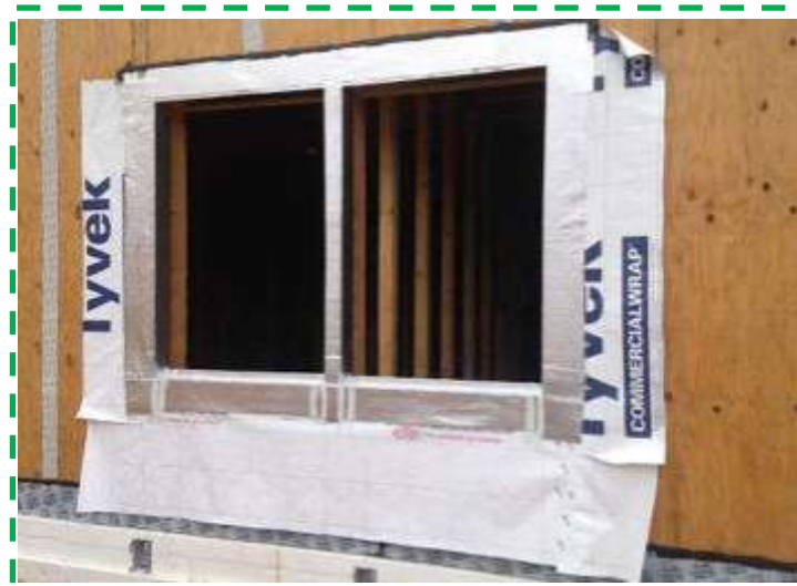
Proper installation sequence, with the housewrap and membrane installed in the rough opening before the window is installed
