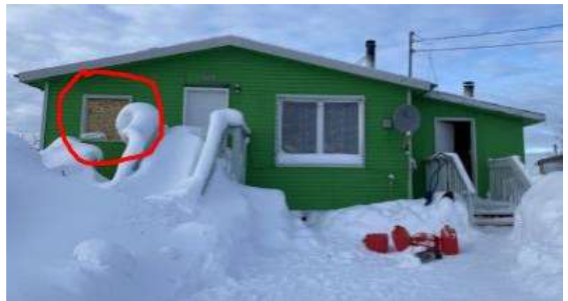
A house in the north with a cracked window boarded over
