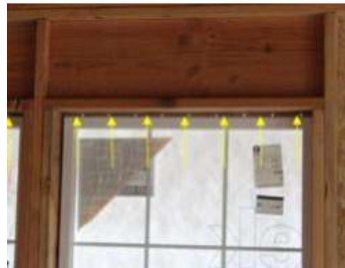
A rough opening gap that is too big at the window head (a big 1" gap)
