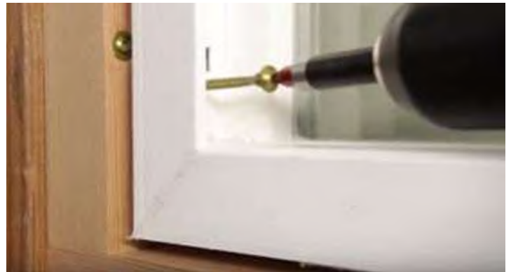
Directly fastening through the window frame can also be overdone.
