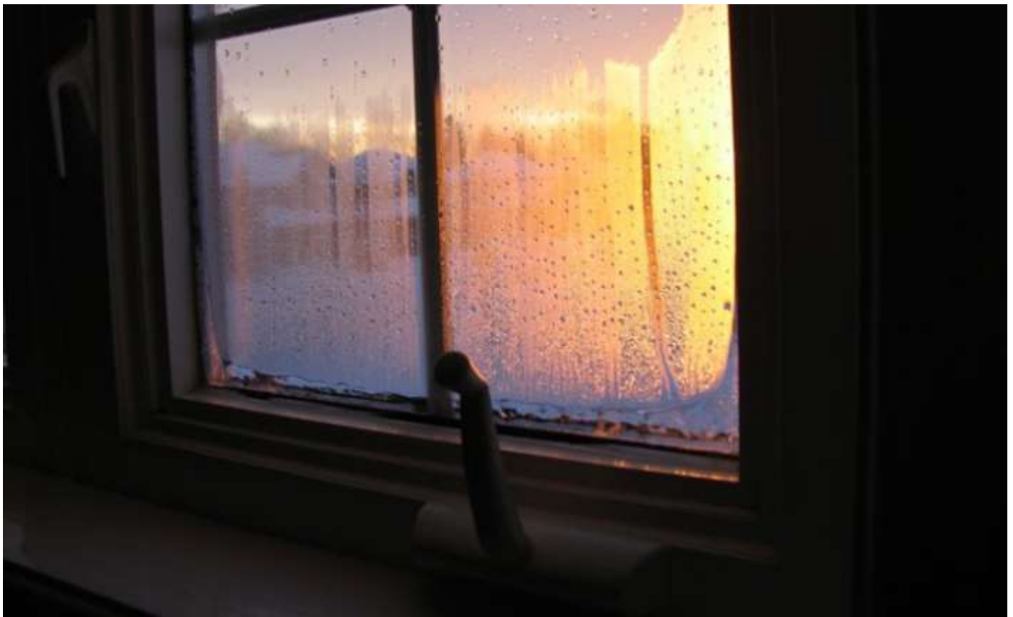
Condensation formation on the interior surface of a window with ice formation along the frame
