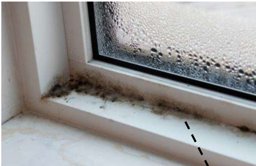
A window with condensation and mould growth
