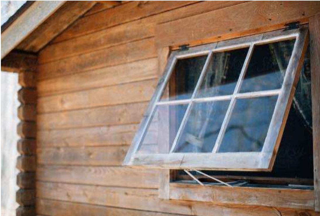
A window left open through the winter to manage overheating
