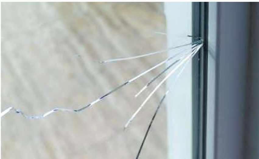
A crack in the glass of the window
