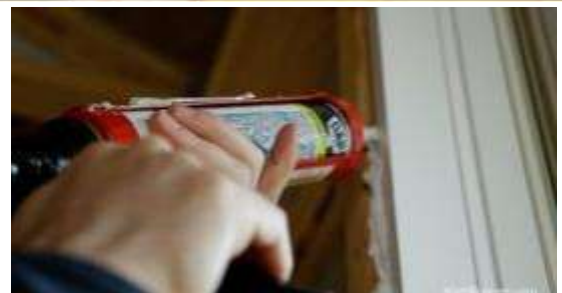
The interior perimeter and rough opening gap being sealed with foam backer rod and sealant
