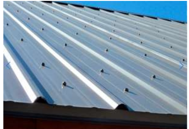
Exposed-fastener metal roofing (lots of fastener holes through the roof)
