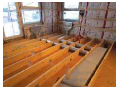
A hot-floor construction in progress with air ducting installed in the service cavity before the flooring is installed over top
