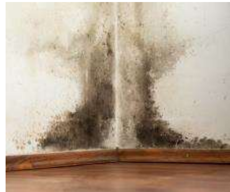
Mould growth on a paper-faced gypsum wall
