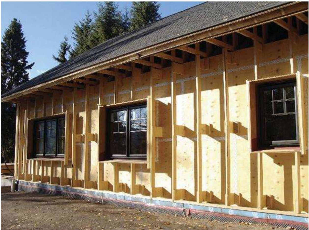
Larsen truss viewed from the outside before insulation and plywood exterior are added
