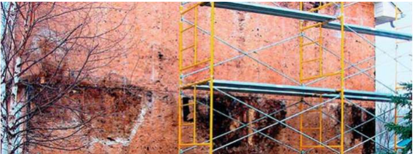
Moisture-damaged wall sheathing due to a discontinuous air barrier at the floor plate
