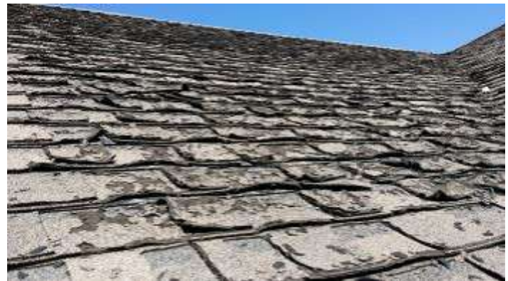
Weathered, sun-damaged roof (three-tab asphalt shingle with organic felt)
