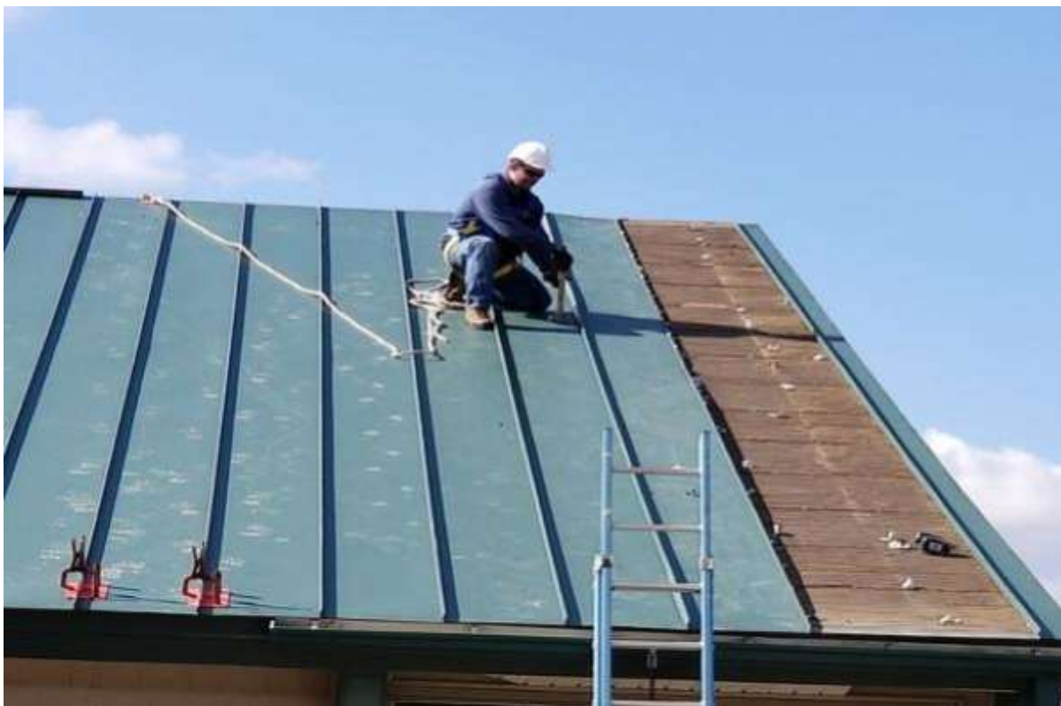
Steel standing-seam roofing panels being installed on a sloped roof. Note that the backup membrane is the full length under the steel roof.
