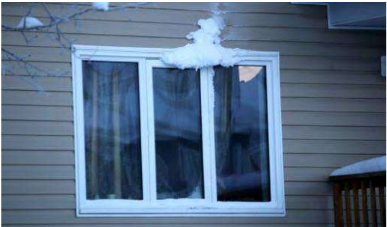
Ice buildup at the window header due to air leakage; warm inside air leaking out through a hole in the air-barrier system (where the wall and window meet)
