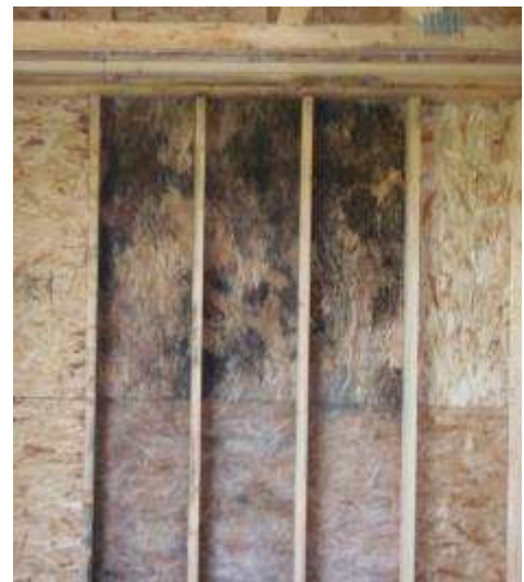
OSB with mould growth in a new house being constructed
