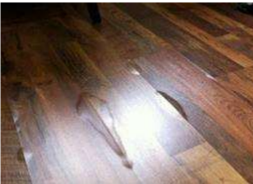
Water-damaged laminate flooring
