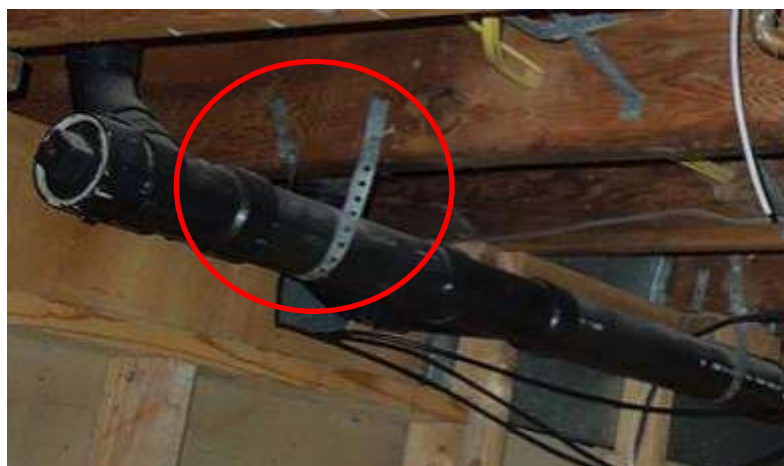
A horizontal pipe supported by a pipe hanger attached to a floor joist
