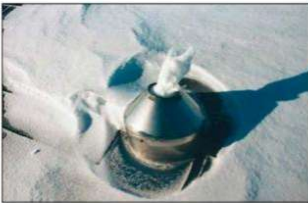
A plumbing vent on a roof blocked with ice
