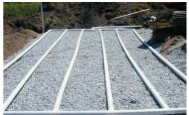
A septic-field installation
