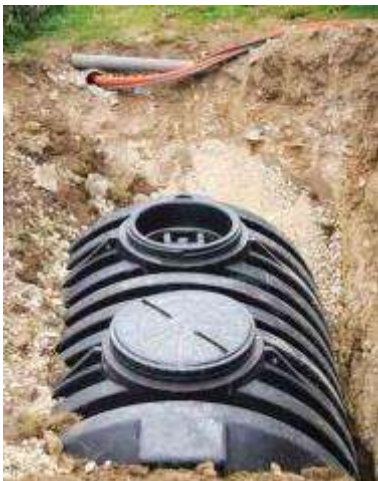
A septic tank
