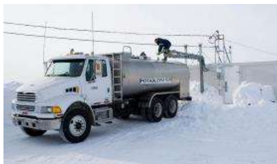
A water truck being filled at a water treatment plant's fill station
