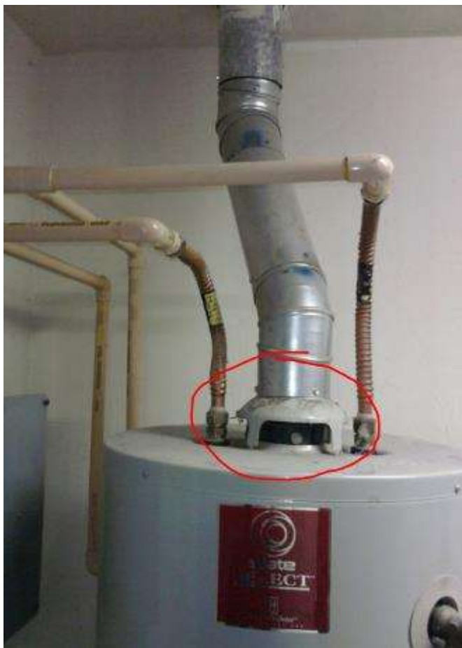
An open draft hood at the top of a hot-water tank circled in red
