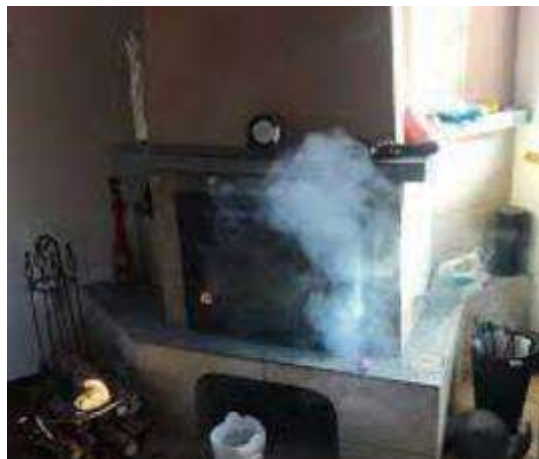
Smoke getting pulled into a house from a wood stove when an exhaust fan is turned on
