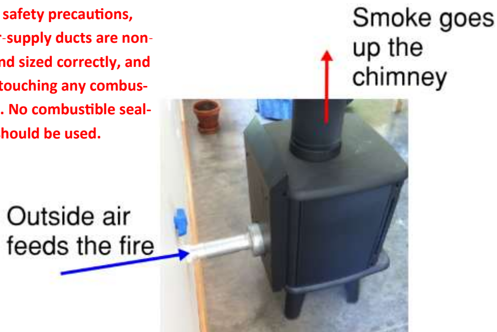
Direct venting of a wood stove with a pipe through the wall
