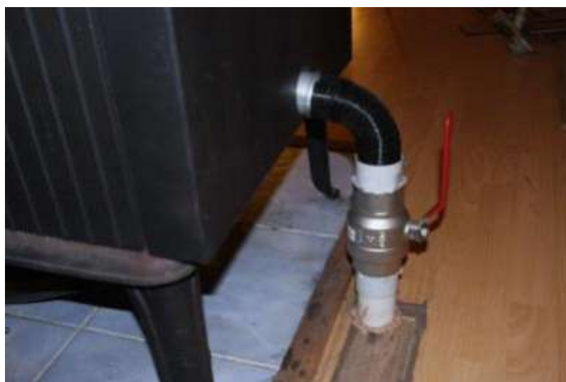
Direct venting of a wood stove with a pipe through the floor and a valve
