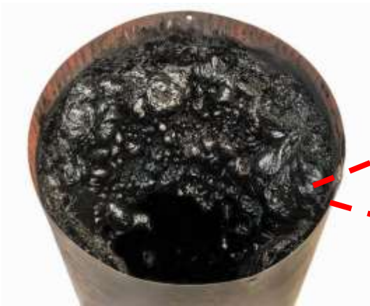
A dangerous creosote build-up in a chimney
